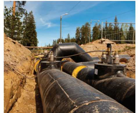
District heating pipeline.
