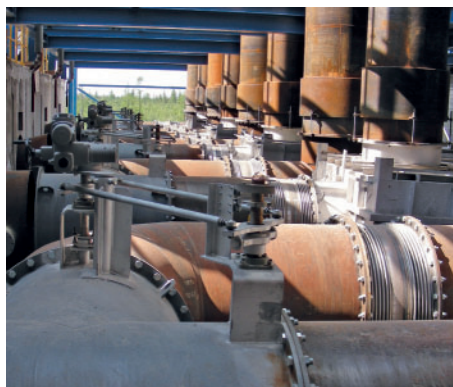
US-types installed in a flue gas system.
